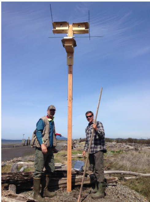
Stan Kostka (left) & Mark Perry (right) install PUMA boxes at Padilla Bay
